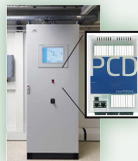
Possible use in primary switch cabinet
