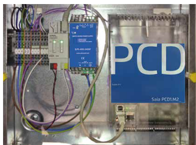
Connection to an existing EIB/KNX installation providing conference rooms with a web connection
