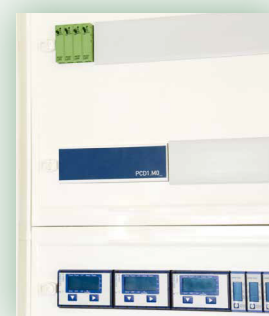
Possible use in an electrical cabinet
